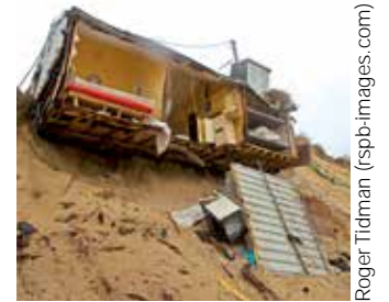
Tidal surge damage on the Norfolk coast, winter 2013
